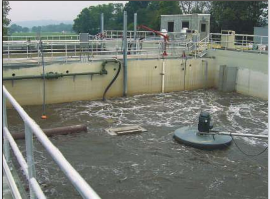
Sequencing Batch Reactor (SBR), Rising Sun, Indiana
